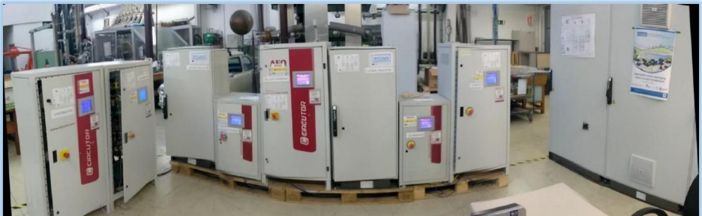
CITCEA-UPC microgrid ready for testing
